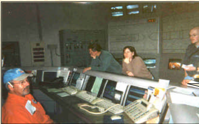
Control Room for Hanging Lake Tunnel
