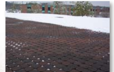
Pavers are largely free from ice and snow and accumulation Photo Courtesy Interlocking Concrete Pavement Institute
