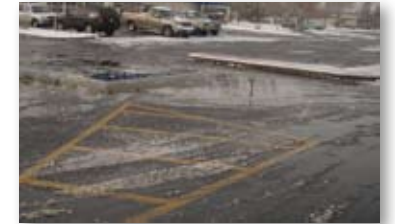
Standing water and free/thaw cycles create and auto and pedestrian hazard and shorten the life of the paving material. Photo by Michelle DeLaria.
