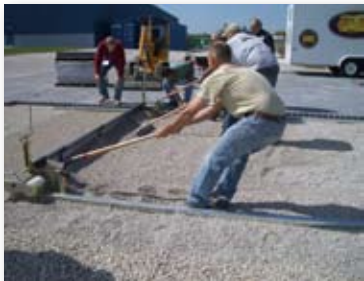
Screed boards are used to lay a level setting bed. Photo by Michelle DeLaria.
