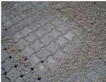
One quarter inch aggregate is swept into the paver joints. Photo by Michelle DeLaria.
