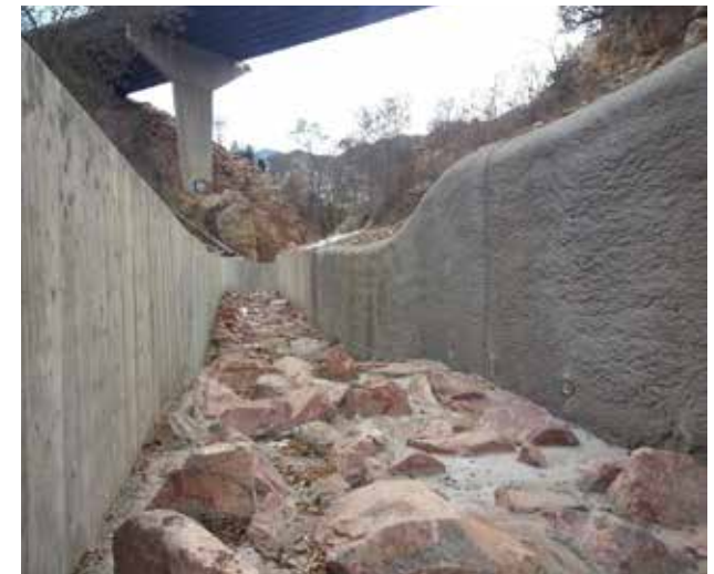
View down the channel constructed as part of Phase 1 in Williams Canyon. A roadway parallel to the channel is above on the left, out of sight. The Highway 24 overpass is visible above.
