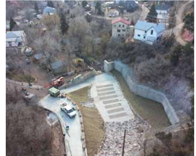
View of the sediment/debris basin under construction as part of Phase 1 of the Williams Canyon project in Manitou Springs. The roadway adjacent to the channel is on the left. The photo is taken from the Highway 24 overpass which crosses Williams Canyon.
