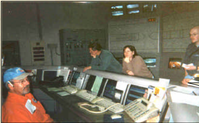
Control Room for Hanging Lake Tunnel
